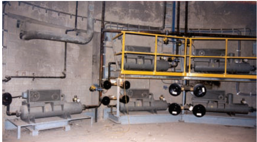
Compact blower arrangements for each sector increase open floor space below the silo floor.
