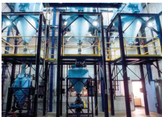
Multi-unit receiving and transfer stations allow full-scale testing and material evaluations.
