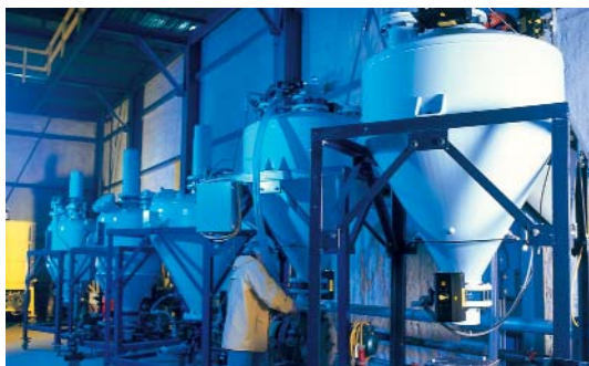
Modular equipment assemblies facilitate test programs
